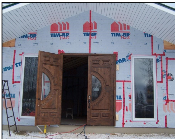
Front doors have been installed in the Keekanaw Multi-Purpose Facility. The MCFN logo has been etched into the windows.
