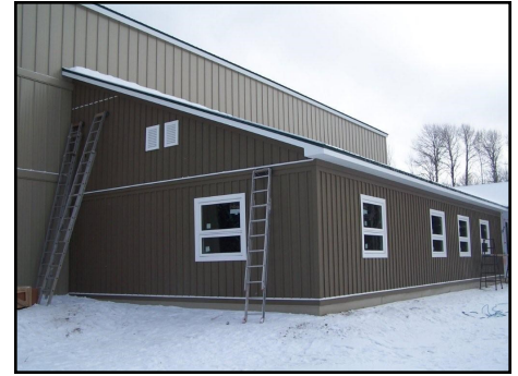
Office wing of the Keekawnaw Multi-Purpose Facility. Interior work will commence in the spring of 2011.
